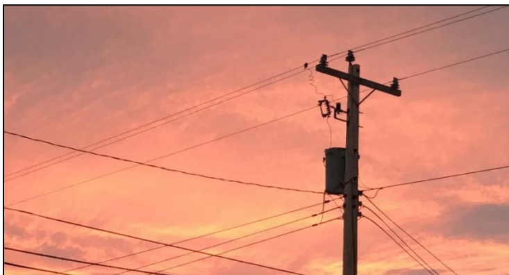
QEC's distribution system sees preventative maintenance in the summer.
