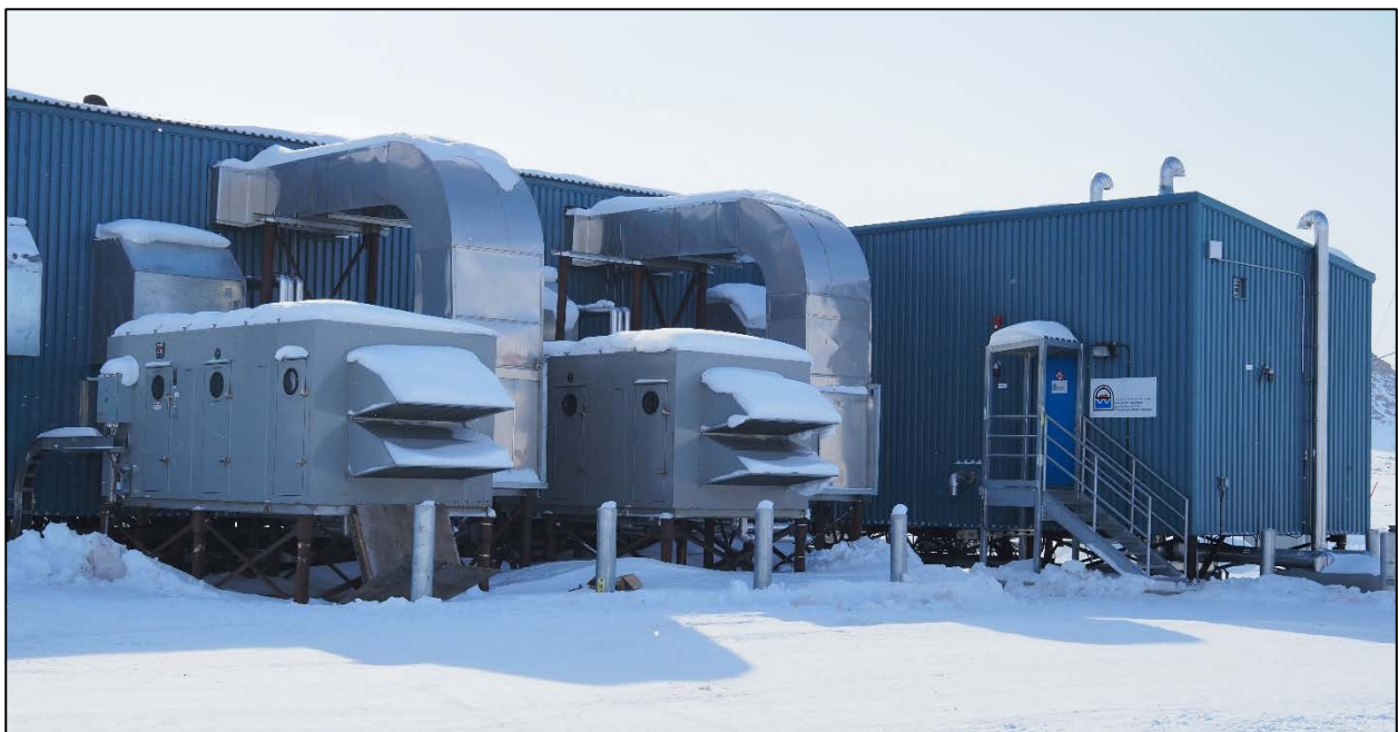
Qikiqtarjuaq's power plant, built in 2016.
