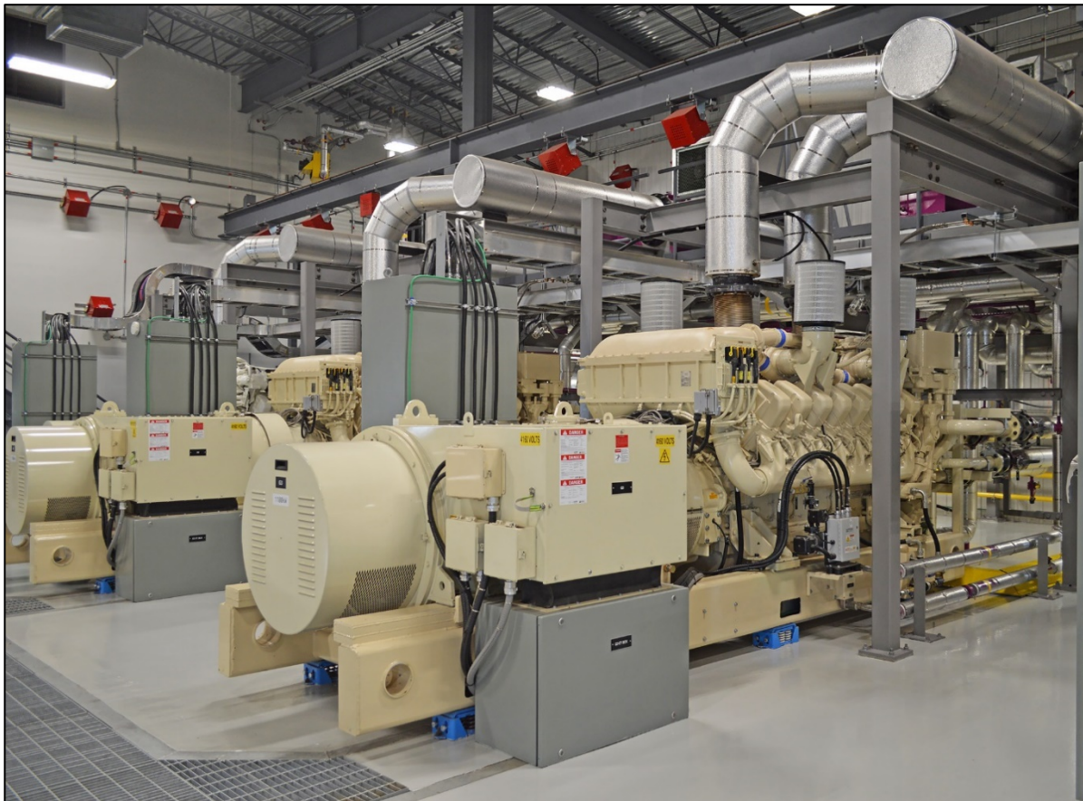
Kinngait power plant, built in 2018.
